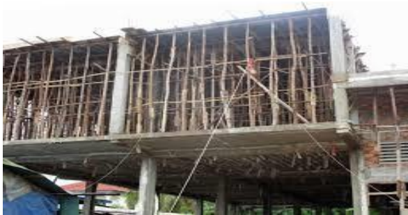
Figure. 1: A building with Floating columns at first storey
